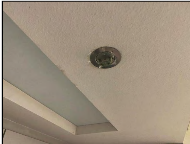
Figure 3: Old sprinkler head to be replaced
