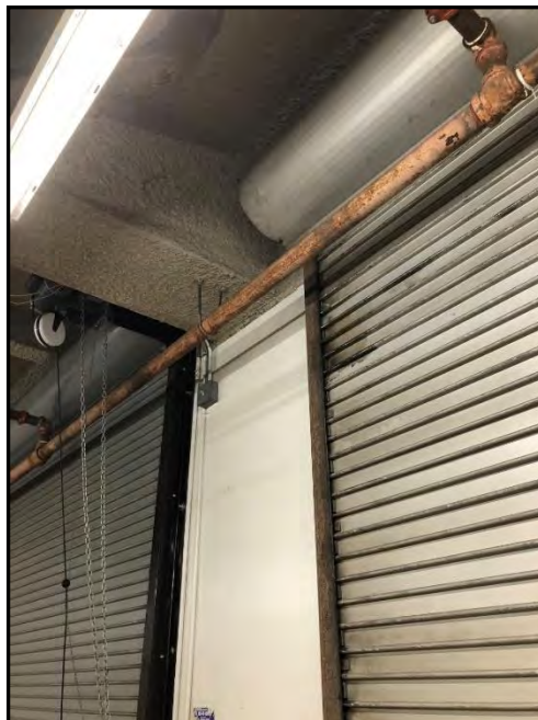
Figure 2: Rusted fire sprinkler piping
