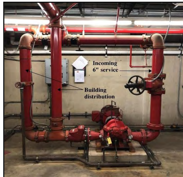
Figure 4: Fire pump room
