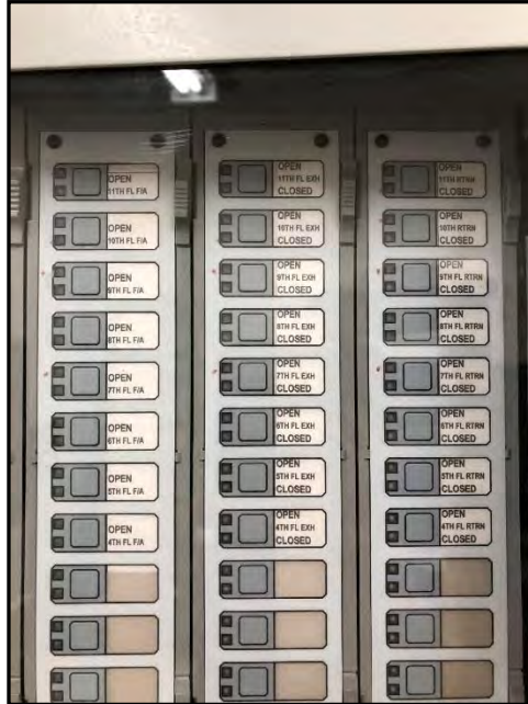
Figure 10: Existing smoke evacuation manual override panel
