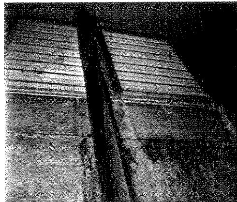
No._9 Hoistway ventilation & guide rail
