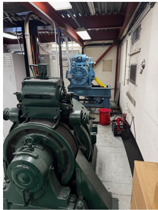
Central Justice Center – Elevators 1 and 2
