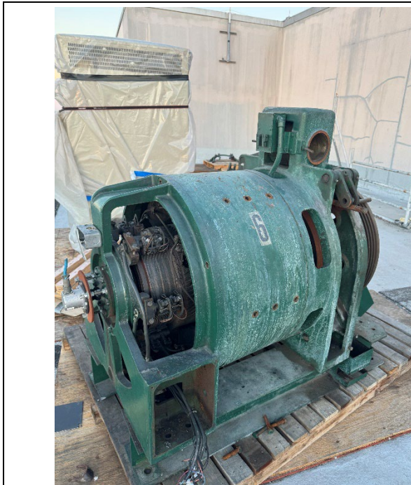
Central Justice Center – Elevator 1
