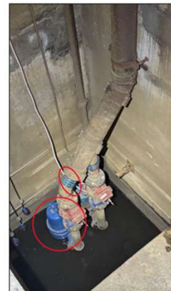
Pump and pipe connector
