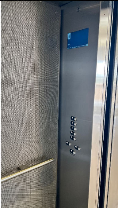
East Los Angeles Courthouse - Elevators
