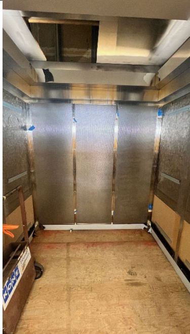
East Los Angeles Courthouse – Elevators
