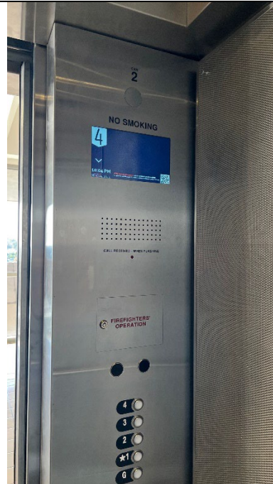
East Los Angeles Courthouse - Elevators
