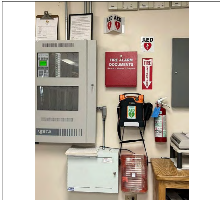
Hayward Hall of Justice – Fire Alarm
