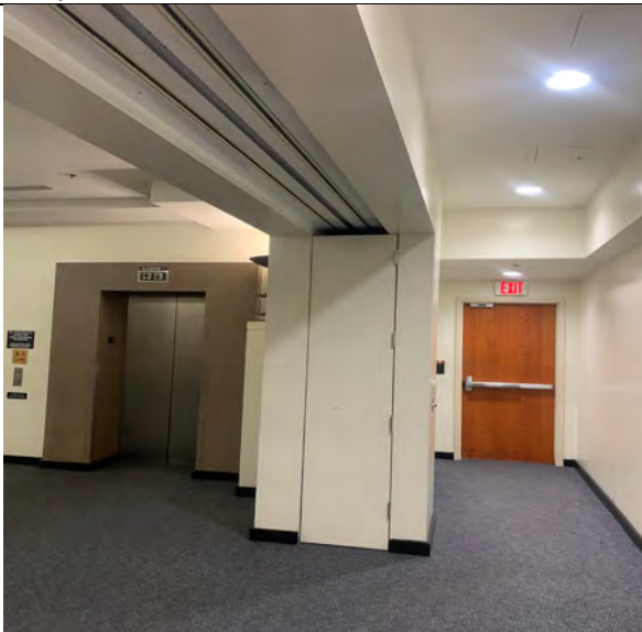
Betty Lou Lamoreaux Justice Center – Fire Alarm
