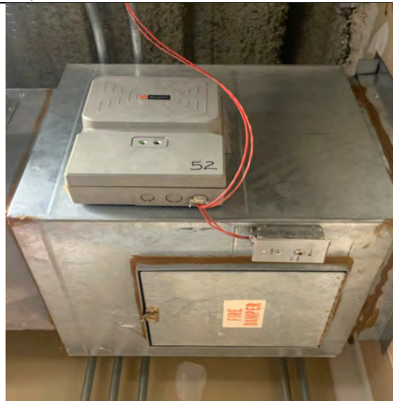
Betty Lou Lamoreaux Justice Center – Fire Alarm
