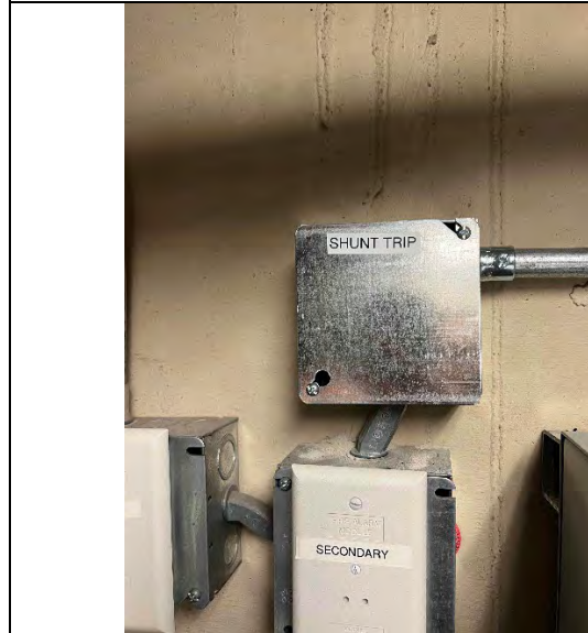
Hayward Hall of Justice - Elevator
