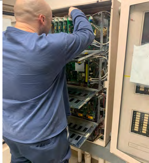
Betty Lou Lamoreaux Justice Center – Fire Alarm
