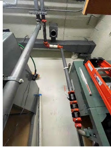
Fremont Hall of Justice - Elevator
