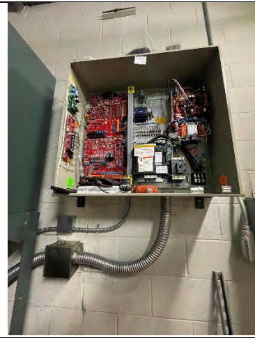
Fremont Hall of Justice - Elevator
