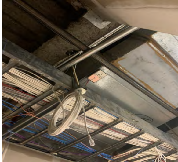
Betty Lou Lamoreaux Justice Center – Fire Alarm
