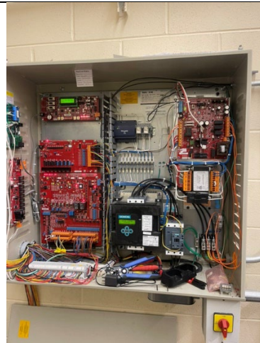
Fremont Hall of Justice - Elevator
