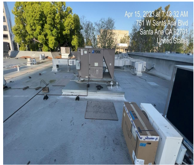
Civil Complex Center – HVAC/BMS
