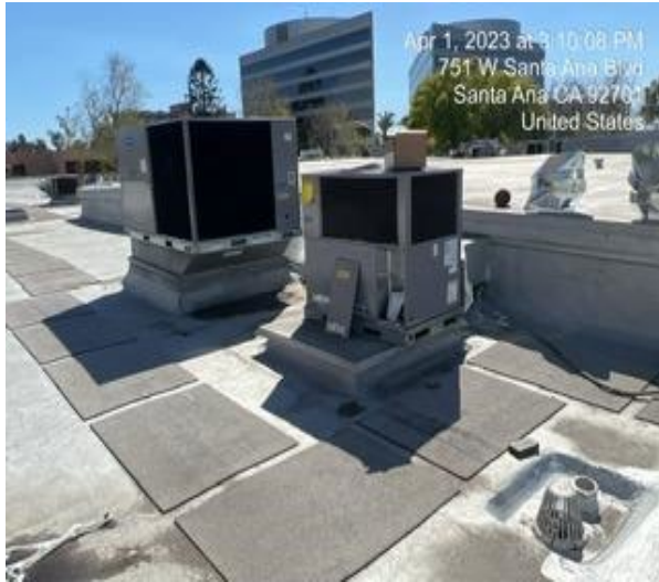
Civil Complex Center – HVAC/BMS
