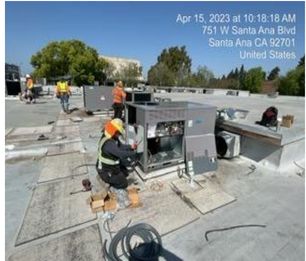
Civil Complex Center – HVAC/BMS
