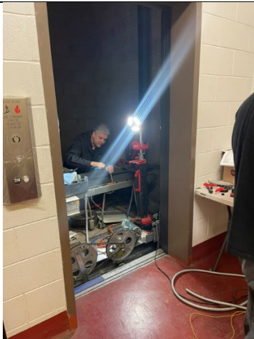
Fremont Hall of Justice - Elevator
