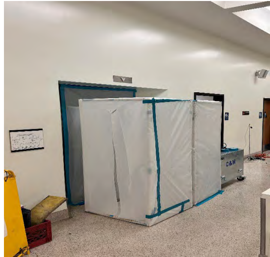
Harbor Justice Center-Newport Beach - Elevators
