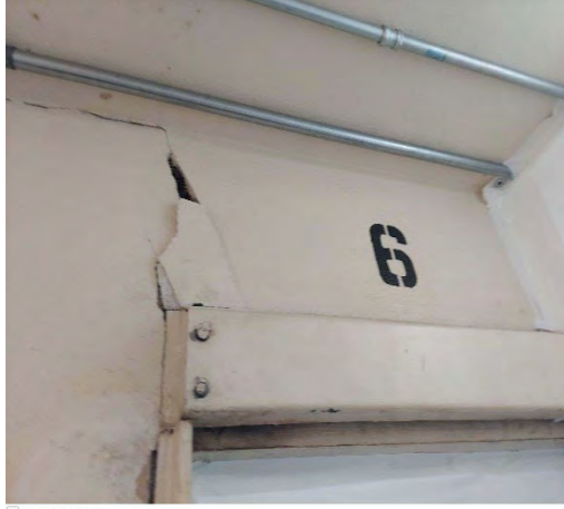
Deteriorated and buckled wall
