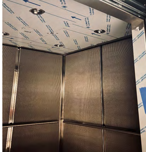
Harbor Justice Center-Newport Beach - Elevators
