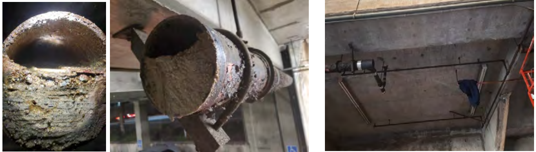
Planter drain lines obstructed with cement
