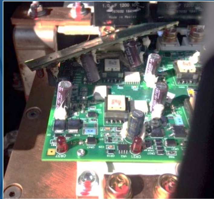
Blown Power Supply
