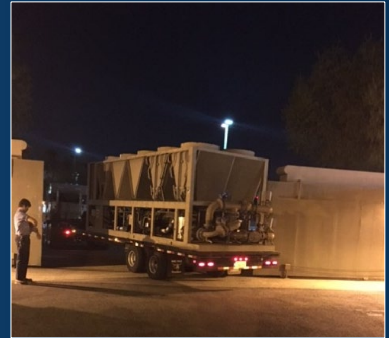
Temporary Chiller Delivery
