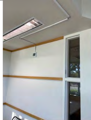
Carol Miller Justice Center Court Facility – Fire Protection
