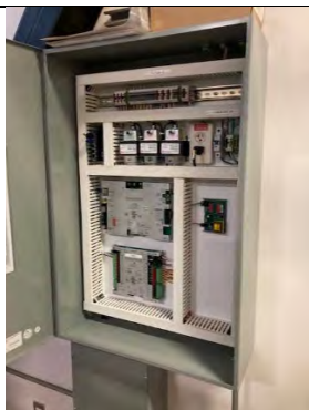
Michael D. Antonovich Antelope Valley Courthouse – Fire Protection
