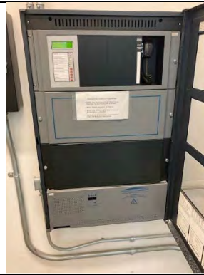
Southwest Justice Center – Fire Protection
