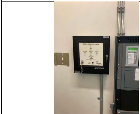
Southwest Justice Center – Fire Protection
