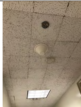
Wiley W. Manuel Courthouse – Fire Protection
