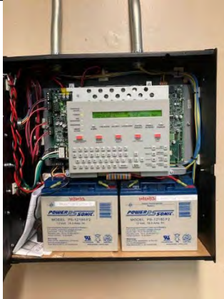
Fresno County Courthouse – Fire Protection
