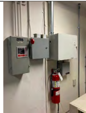
Southwest Justice Center – Fire Protection
