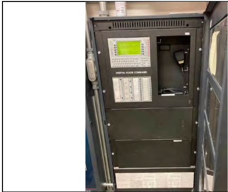
Southwest Justice Center – Fire Protection
