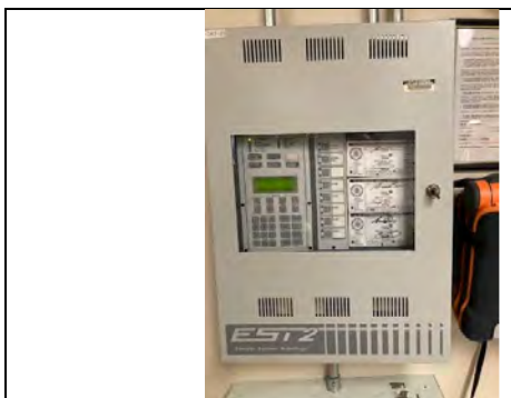
Hayward Hall of Justice – Fire Protection
