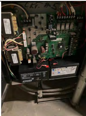
Pomona Courthouse South – Fire Protection
