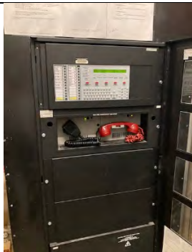
Wiley W. Manuel Courthouse – Fire Protection
