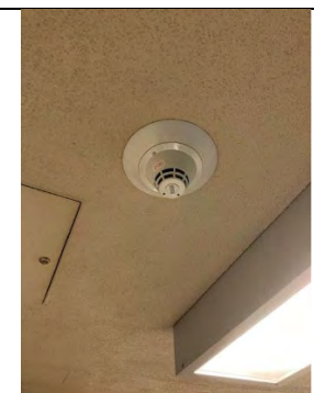
Hayward Hall of Justice – Fire Protection
