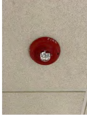
Carol Miller Justice Center Court Facility – Fire Protection
