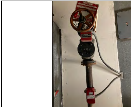
Wiley W. Manuel Courthouse – Fire Protection
