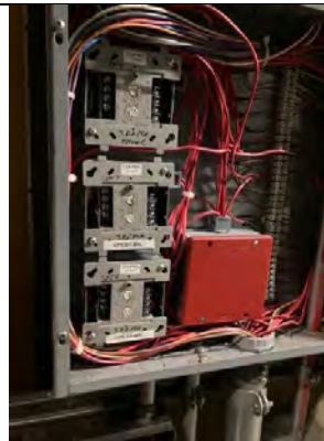
Pomona Courthouse South – Fire Protection
