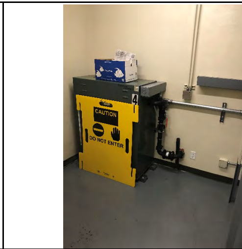
North Justice Center - Elevator 4
