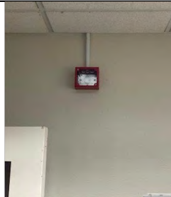
Carol Miller Justice Center Court Facility – Fire Protection
