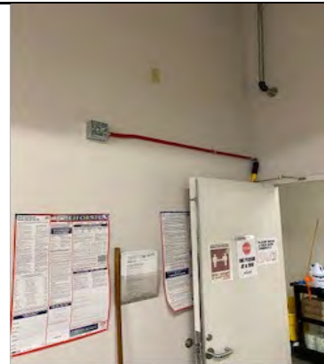
Carol Miller Justice Center Court Facility – Fire Protection
