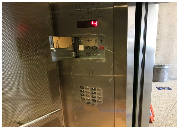
Torrance Courthouse – LA – Elevator
