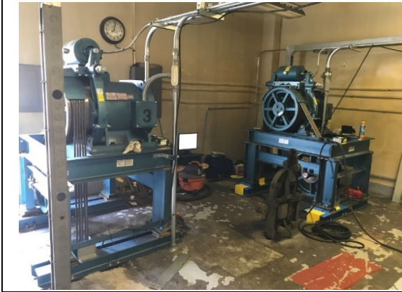
Beverly Hills Courthouse – LA – Elevator
