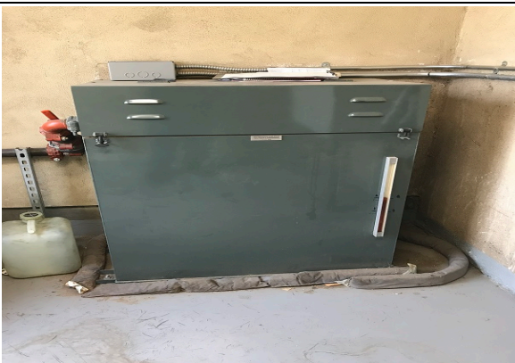
Barstow Courthouse – San Bernardino – Elevator
