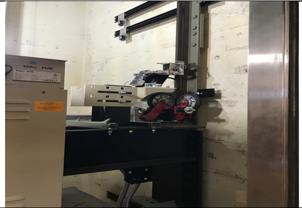
Torrance Courthouse – LA – Elevator
