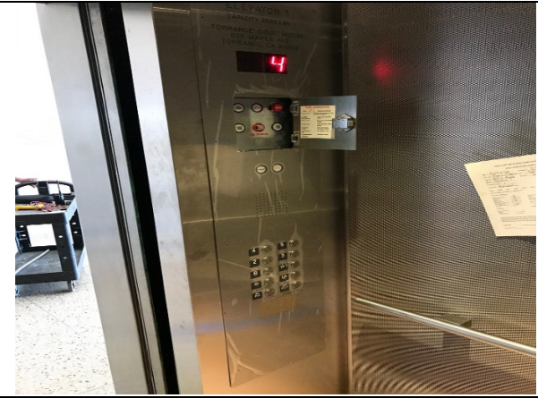
Torrance Courthouse – LA – Elevator
