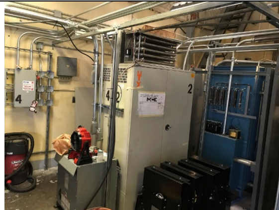
Beverly Hills Courthouse – LA – Elevator
