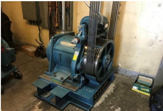
Beverly Hills Courthouse – LA – Elevator
