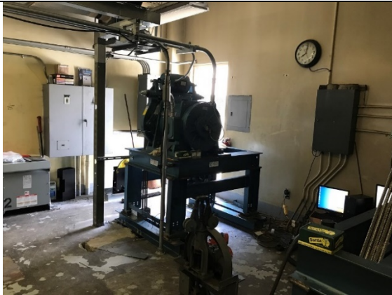
Beverly Hills Courthouse – LA – Elevator
