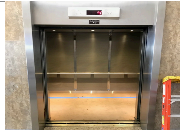
Torrance Courthouse – LA – Elevator
