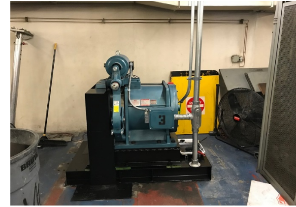
Torrance Courthouse – LA – Elevator
