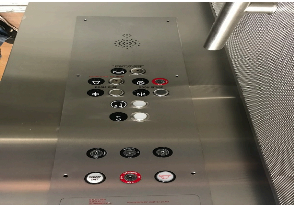
Barstow Courthouse – San Bernardino – Elevator
