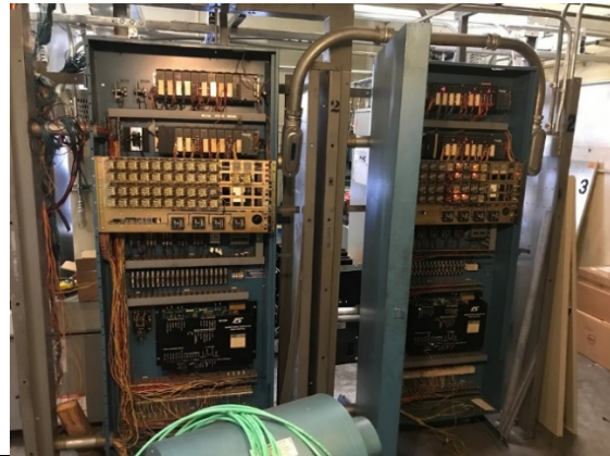
Beverly Hills Courthouse – LA – Elevator
