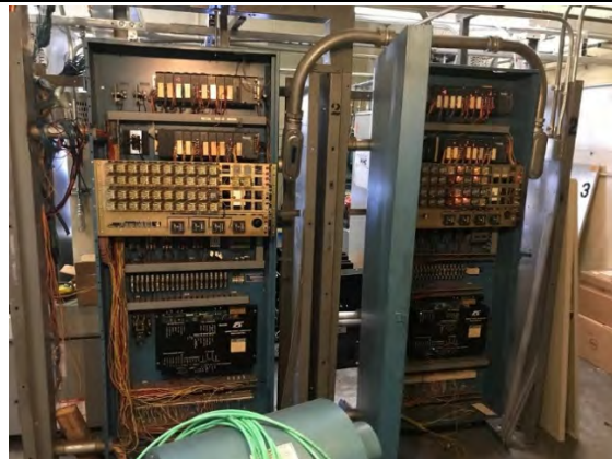
Beverly Hills Courthouse – LA – Elevator
