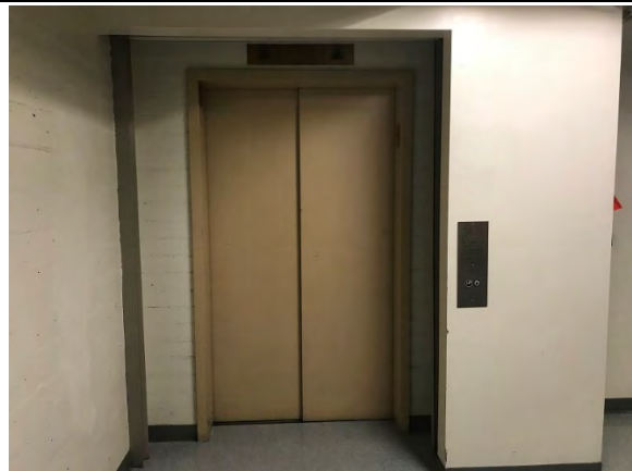
Burbank Courthouse – LA – Elevator
