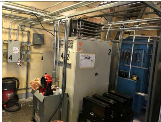
Beverly Hills Courthouse – LA – Elevator
