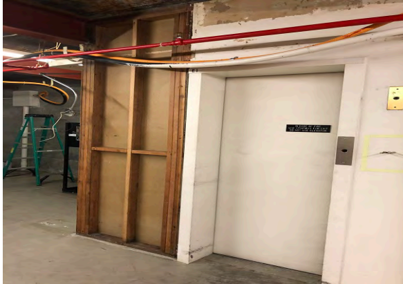
Northern Branch Courthouse – San Mateo – Elevator
