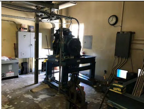
Beverly Hills Courthouse – LA – Elevator
