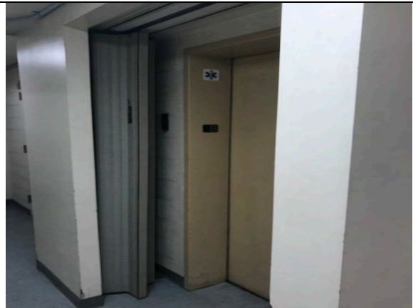
Burbank Courthouse – LA – Elevator
