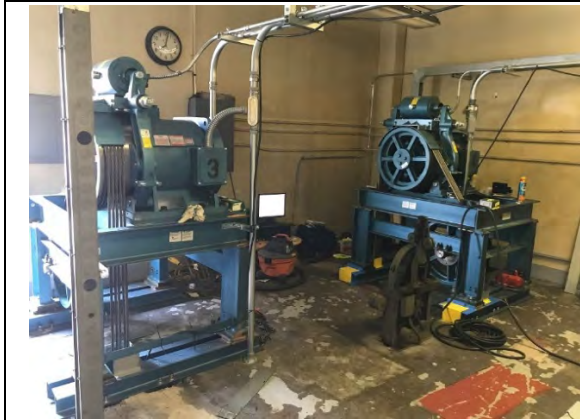
Beverly Hills Courthouse – LA – Elevator
