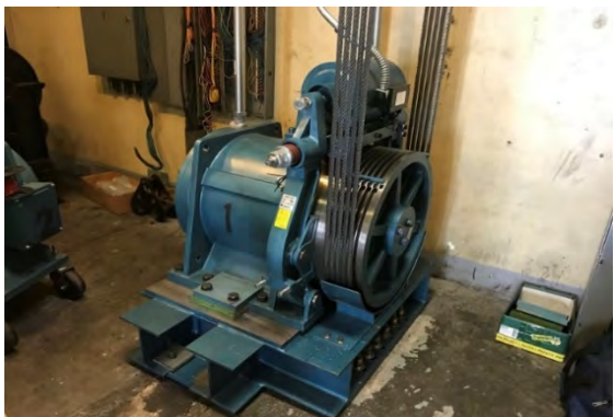
Beverly Hills Courthouse – LA – Elevator
