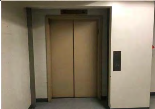
Burbank Courthouse - LA - Elevator
