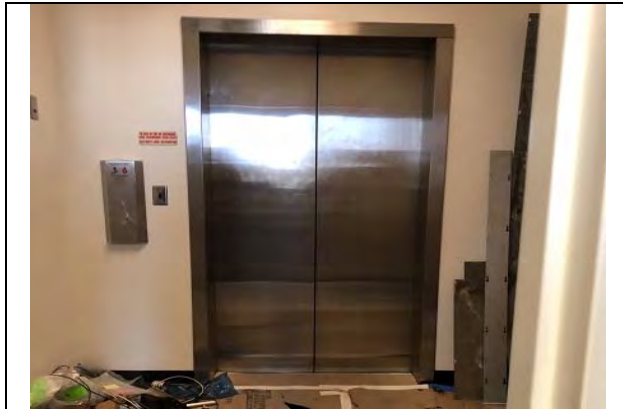
Inglewood Courthouse - LA - Elevator
