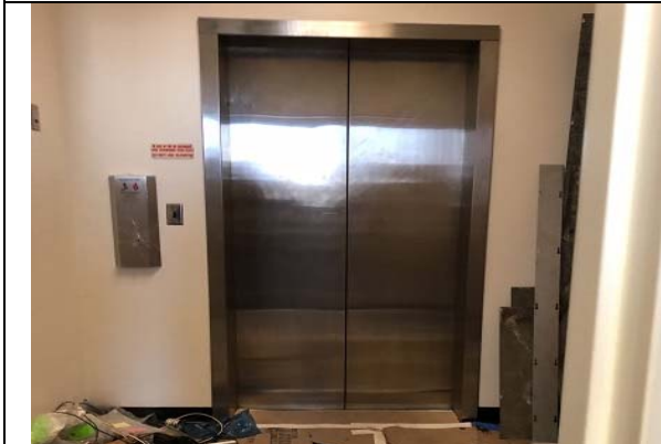
Inglewood Courthouse - LA - Elevator
