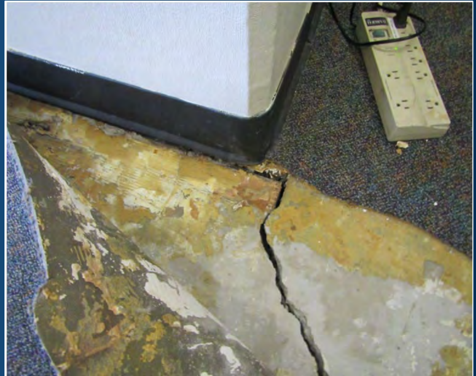
Cracked slab on grade in Jury Assembly Room
