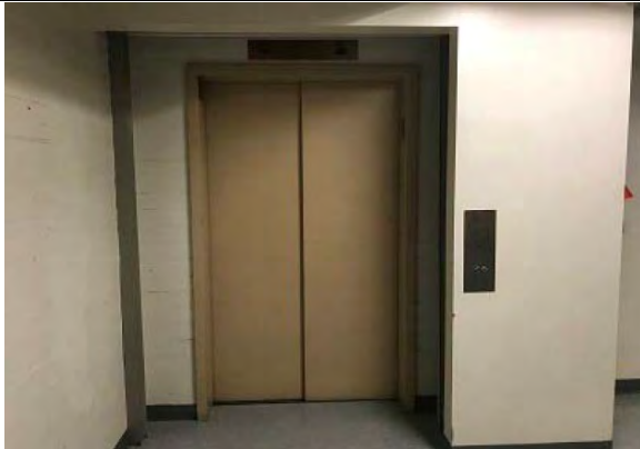
Burbank Courthouse - LA - Elevator
