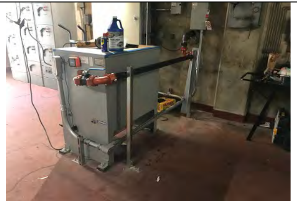
Inglewood Juvenile Courthouse - LA - Elevator
