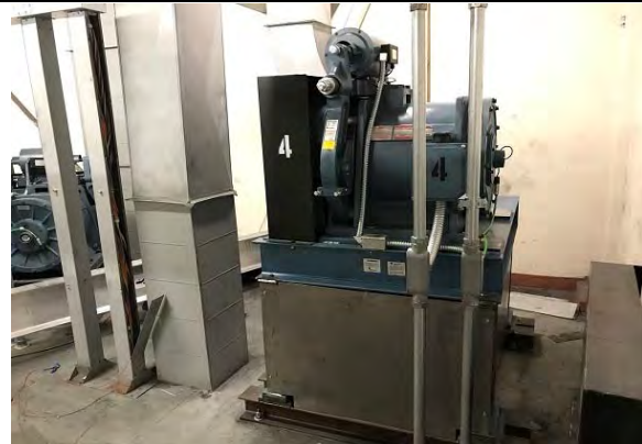
Alhambra Courthouse - LA - Elevator
