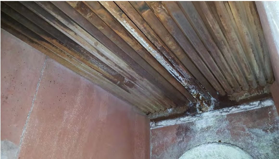
Above: Existing boiler with corroded and leaking tubes. (top photos) Below: Boiler with newly replaced tubes. (bottom photo)
