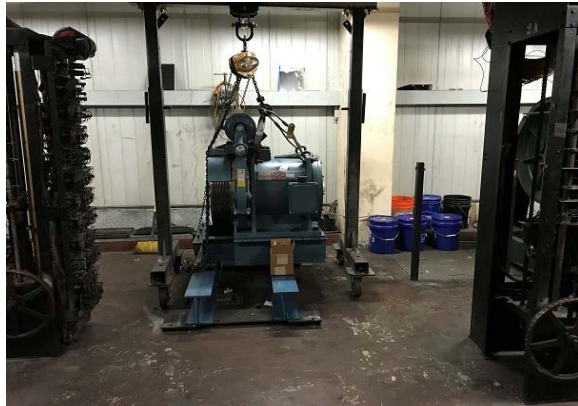
Inglewood Courthouse – LA - Elevator
