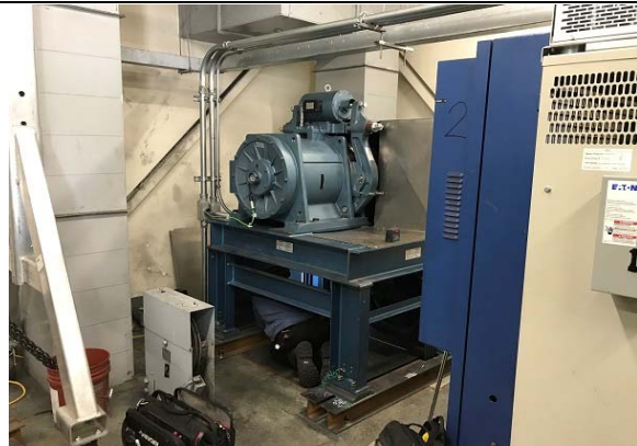
Alhambra Courthouse - LA - Elevator
