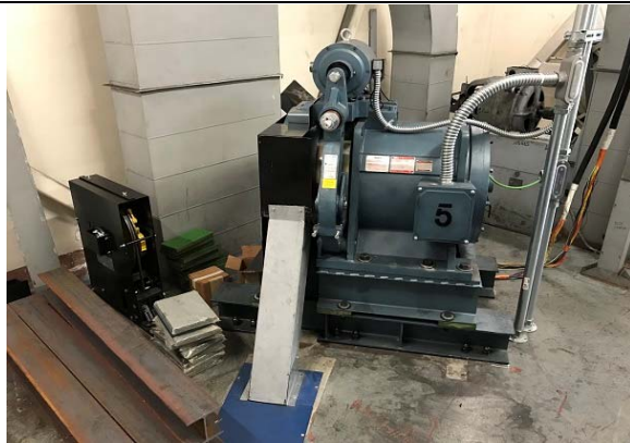
Alhambra Courthouse - LA - Elevator
