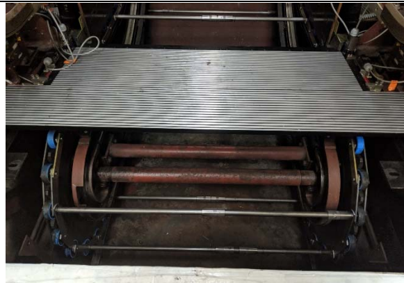
Stanley Mosk Courthouse - LA - Escalators Phase 7
