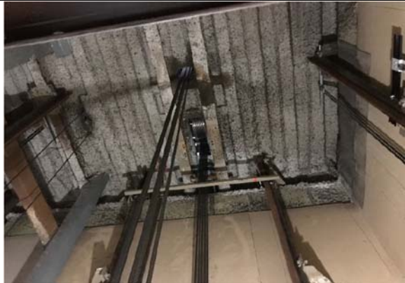
Edelman Children's Court - LA - Elevator
