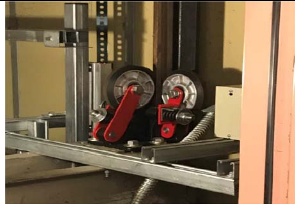
Edelman Children's Court - LA - Elevator
