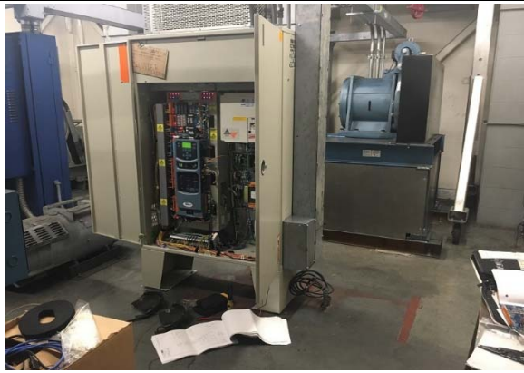
Alhambra Courthouse - LA - Elevator
