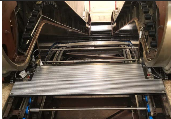
Stanley Mosk Courthouse - LA - Escalators Phase 5
