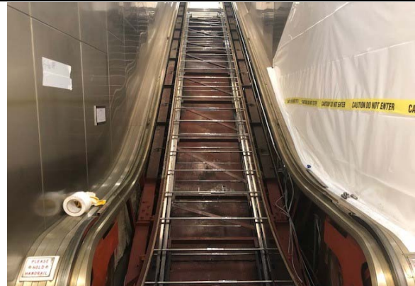
Stanley Mosk Courthouse - LA - Escalators Phase 5
