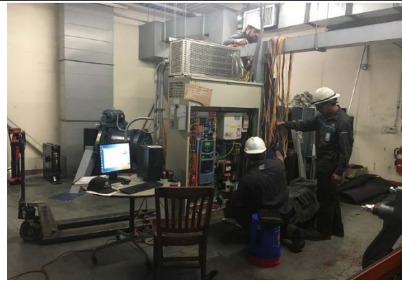
Alhambra Courthouse - LA - Elevator
