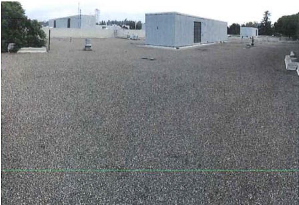
Above: Old roof with 2-4 ply gravel flood coat. Below: Newly replaced roof with Class A 80 mil PVC single-ply membrane
