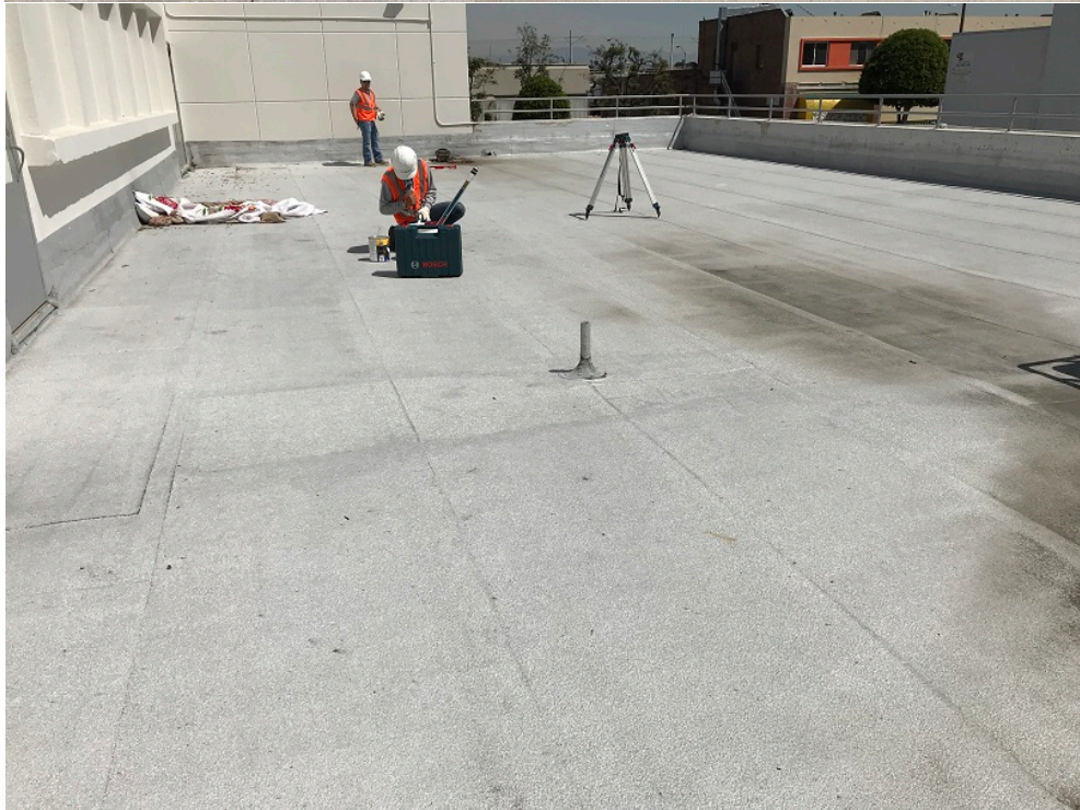
Above: Previous failing built up roof of Inglewood Justice Center Below: Newly replaced SBS multi-ply roof with new building metal & roof drain caps
