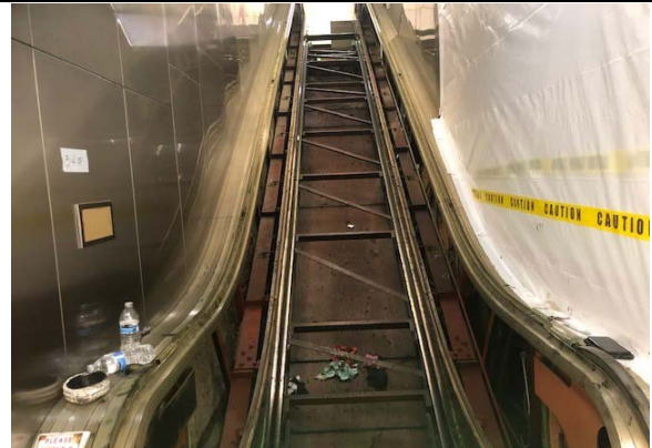
Stanley Mosk Courthouse - LA - Escalators Phase 4
