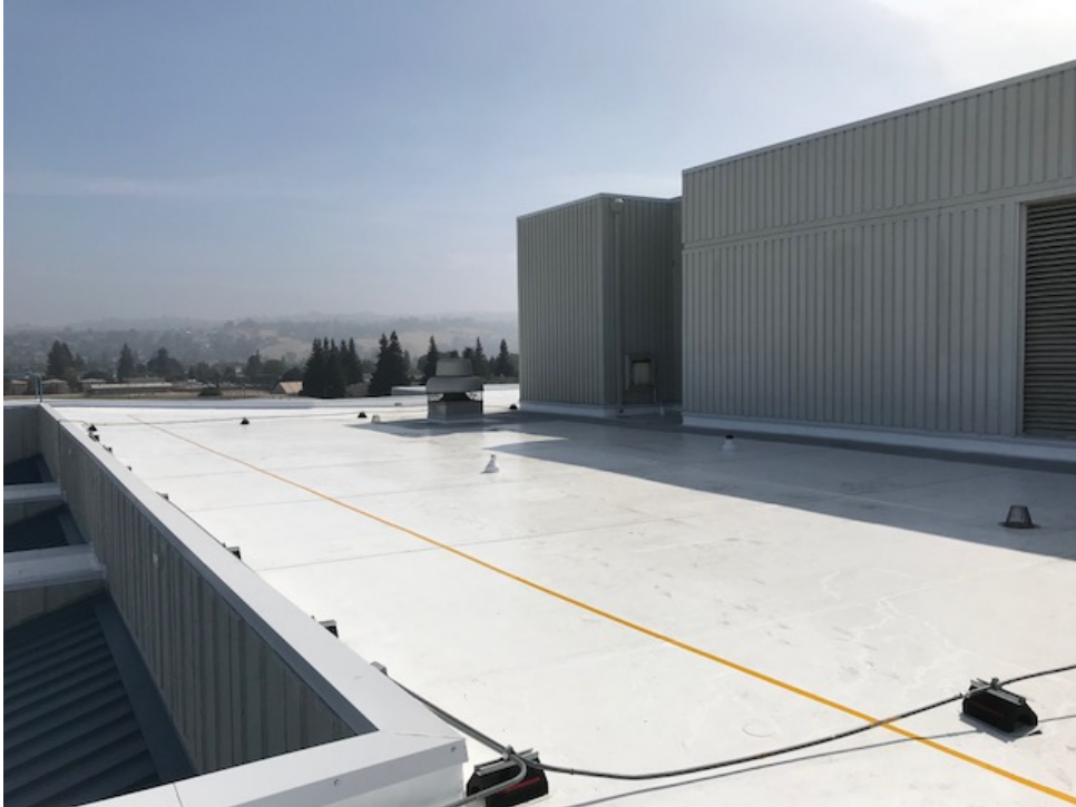
Priority 2: Roof replacement, Bakersfield Juvenile Center, Kern County
