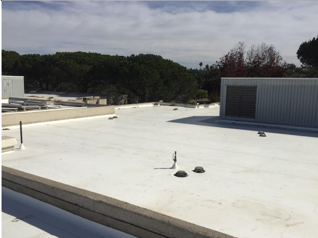
Priority 2: Roof replacement, Hall of Justice - East, Santa Clara County
