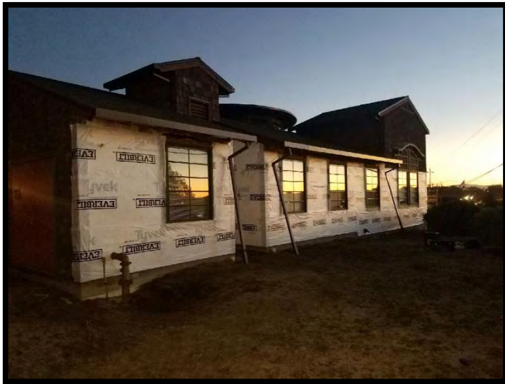
Above: Installation of new weather barrier at the exterior of the courthouse. Below: Courthouse with the installation of new weather tight exterior siding.
