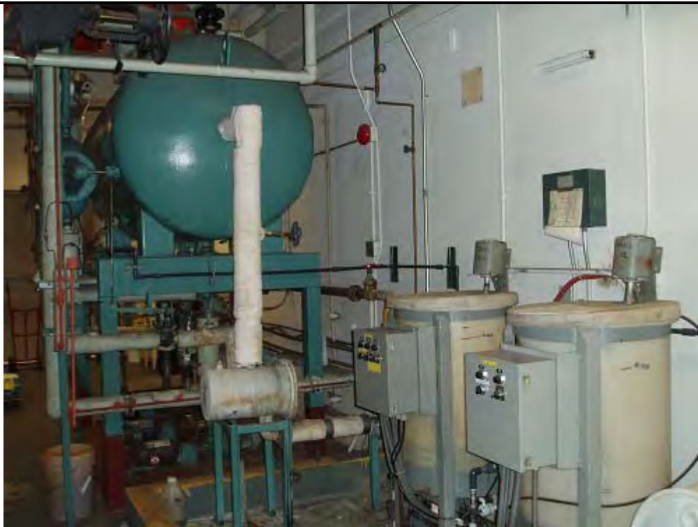
PHOTOGRAPH 1 DESCRIPTION: Boiler Chemical Treatment Area Date: 10 July 2007 ERM 220 West Broadway San Diego, CA
