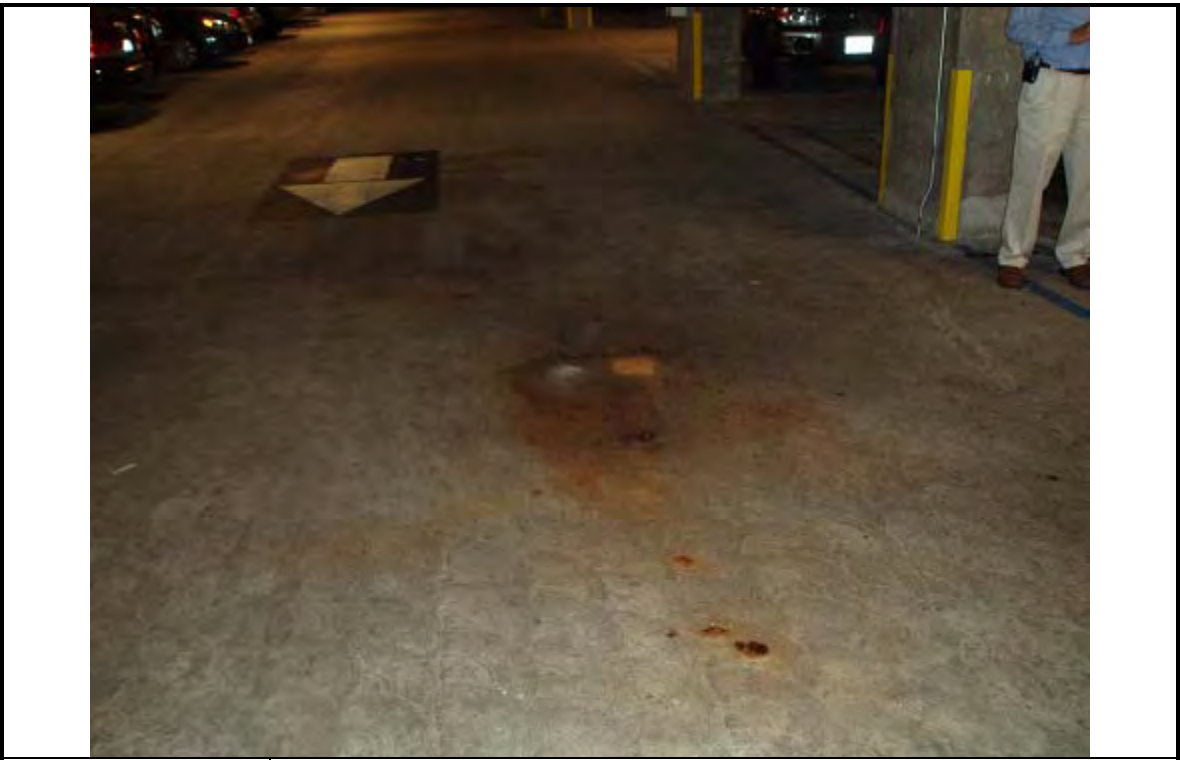
PHOTOGRAPH 11 DESCRIPTION: Parking Garage Drive Aisle Date: 10 July 2007 ERM 330 West Broadway San Diego, CA
