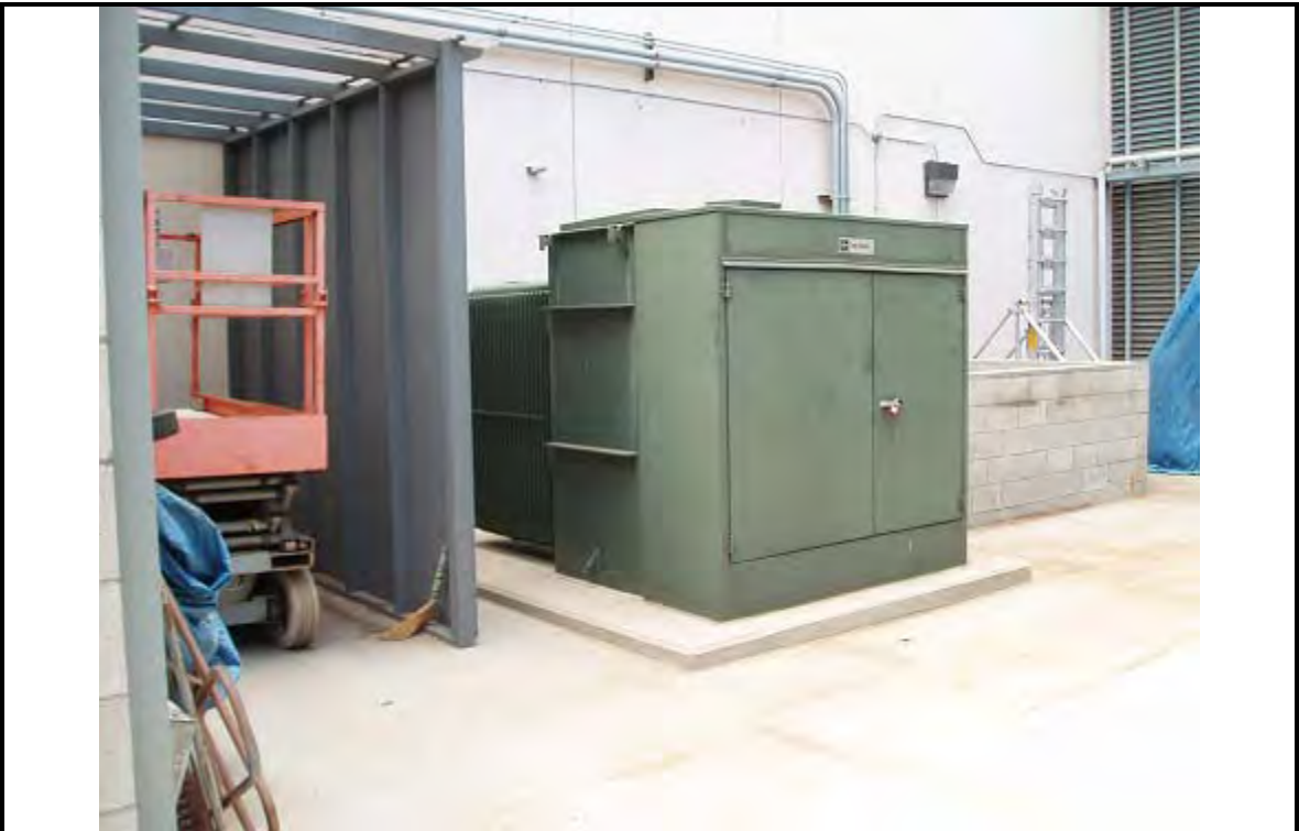
PHOTOGRAPH 5 DESCRIPTION: Transformers at Cooling Tower Date: 10 July 2007 ERM 220 West Broadway San Diego, CA
