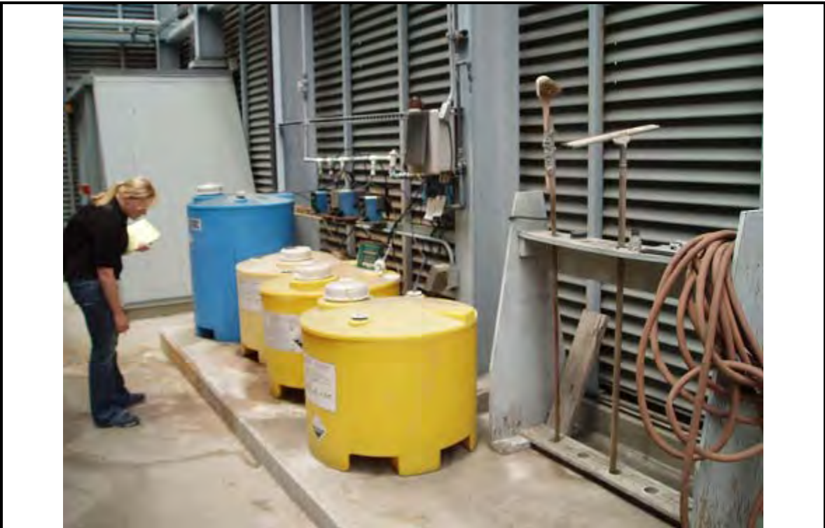
PHOTOGRAPH 4 DESCRIPTION: Cooling Tower Chemical Treatment Area Date: 10 July 2007 ERM 220 West Broadway San Diego, CA
