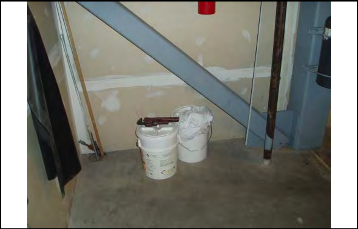
PHOTOGRAPH 3 DESCRIPTION: Boiler Room – Treatment Chemicals Date: 10 July 2007 ERM 330 West Broadway San Diego, CA
