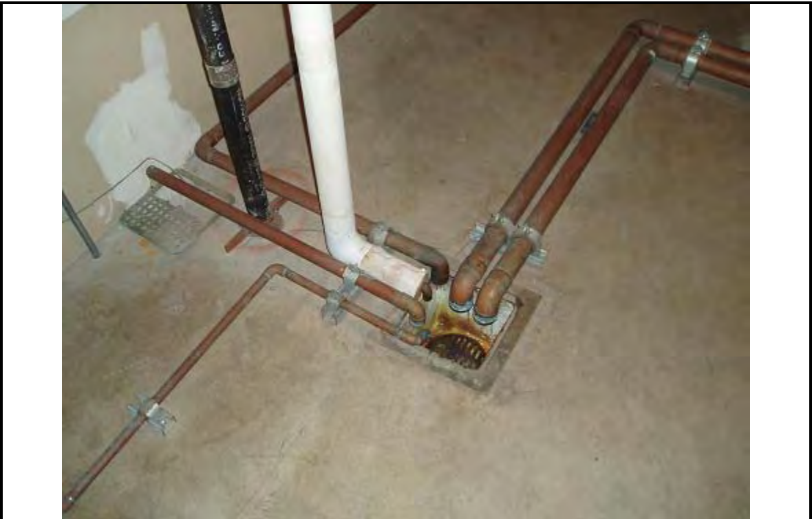
PHOTOGRAPH 4 DESCRIPTION: Boiler Room – Floor Drain Date: 10 July 2007 ERM 330 West Broadway San Diego, CA
