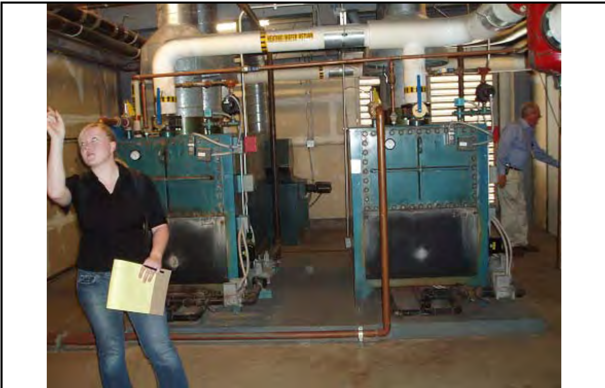
PHOTOGRAPH 2 DESCRIPTION: Boiler Room - Boilers Date: 10 July 2007 ERM 330 West Broadway San Diego, CA
