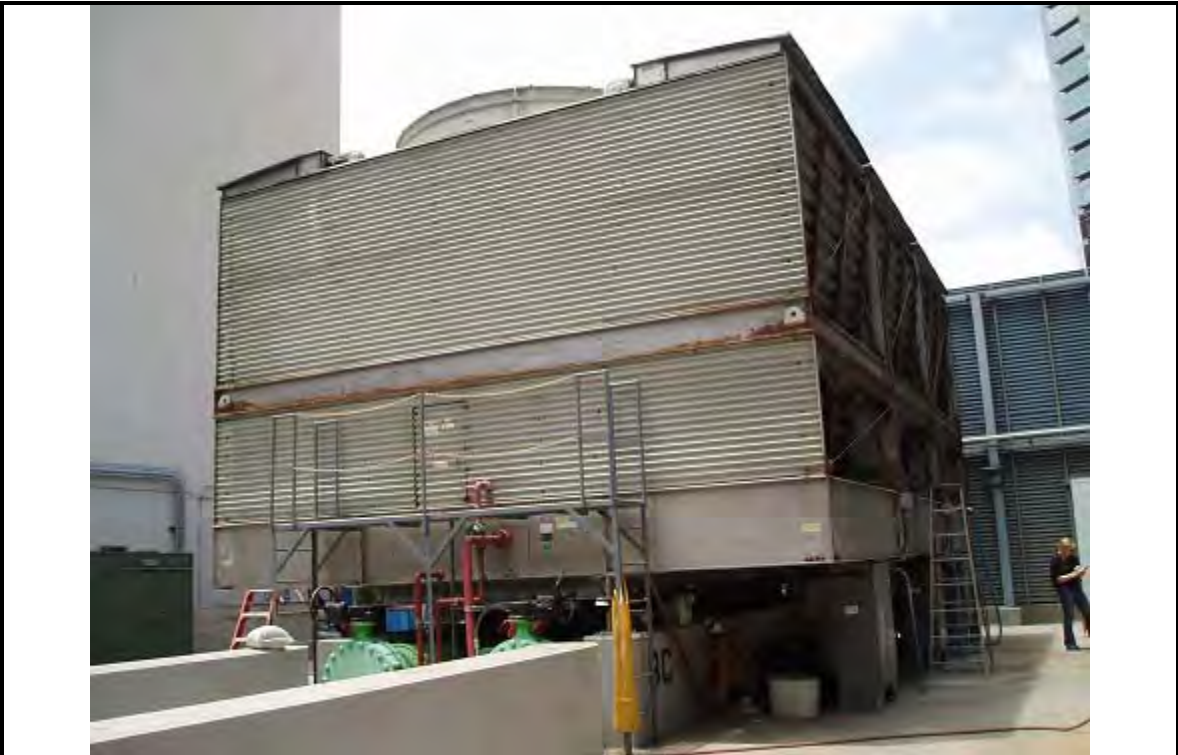
PHOTOGRAPH 3 DESCRIPTION: Cooling Tower Date: 10 July 2007 ERM 220 West Broadway San Diego, CA
