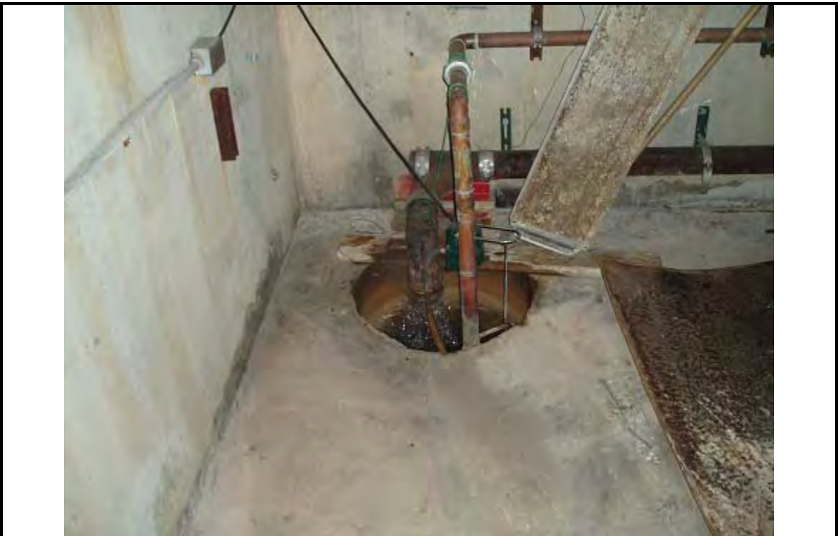
PHOTOGRAPH 6 DESCRIPTION: Cooling Tower Bleed Water Date: 10 July 2007 ERM 220 West Broadway San Diego, CA
