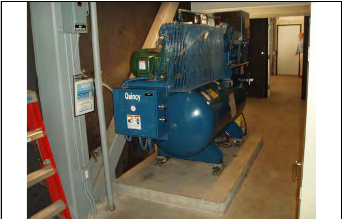
PHOTOGRAPH 5 | DESCRIPTION: Air Compressor
