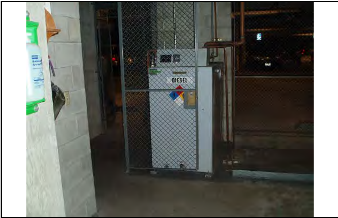
PHOTOGRAPH 9 | DESCRIPTION: Parking Garage Level Two - Emergency Diesel Holding Tank
