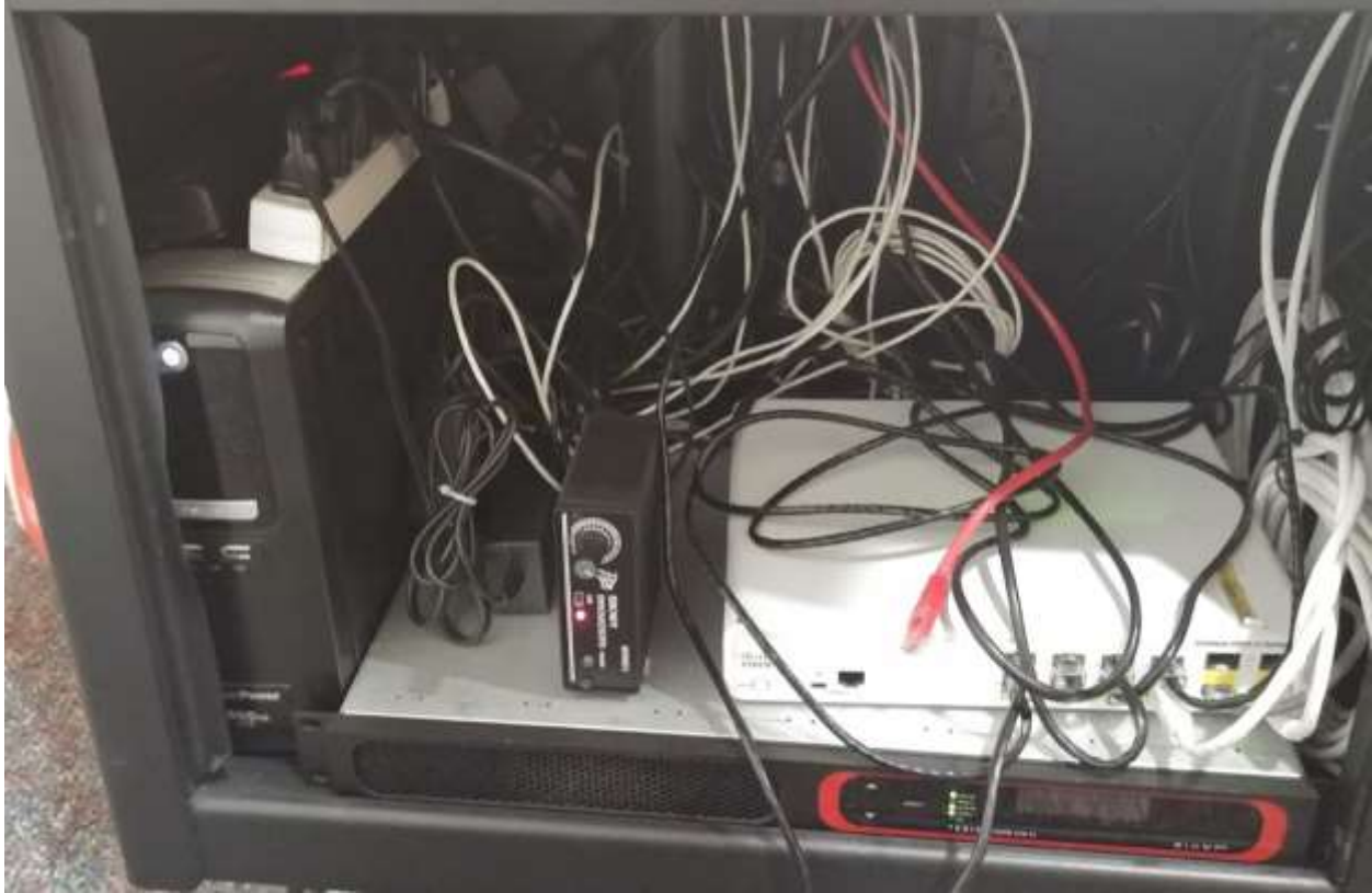
View of inside the media cart. Equipment from left to right: UPS, Biamp DSP, separate sound amplifier, Cisco networking switch.
