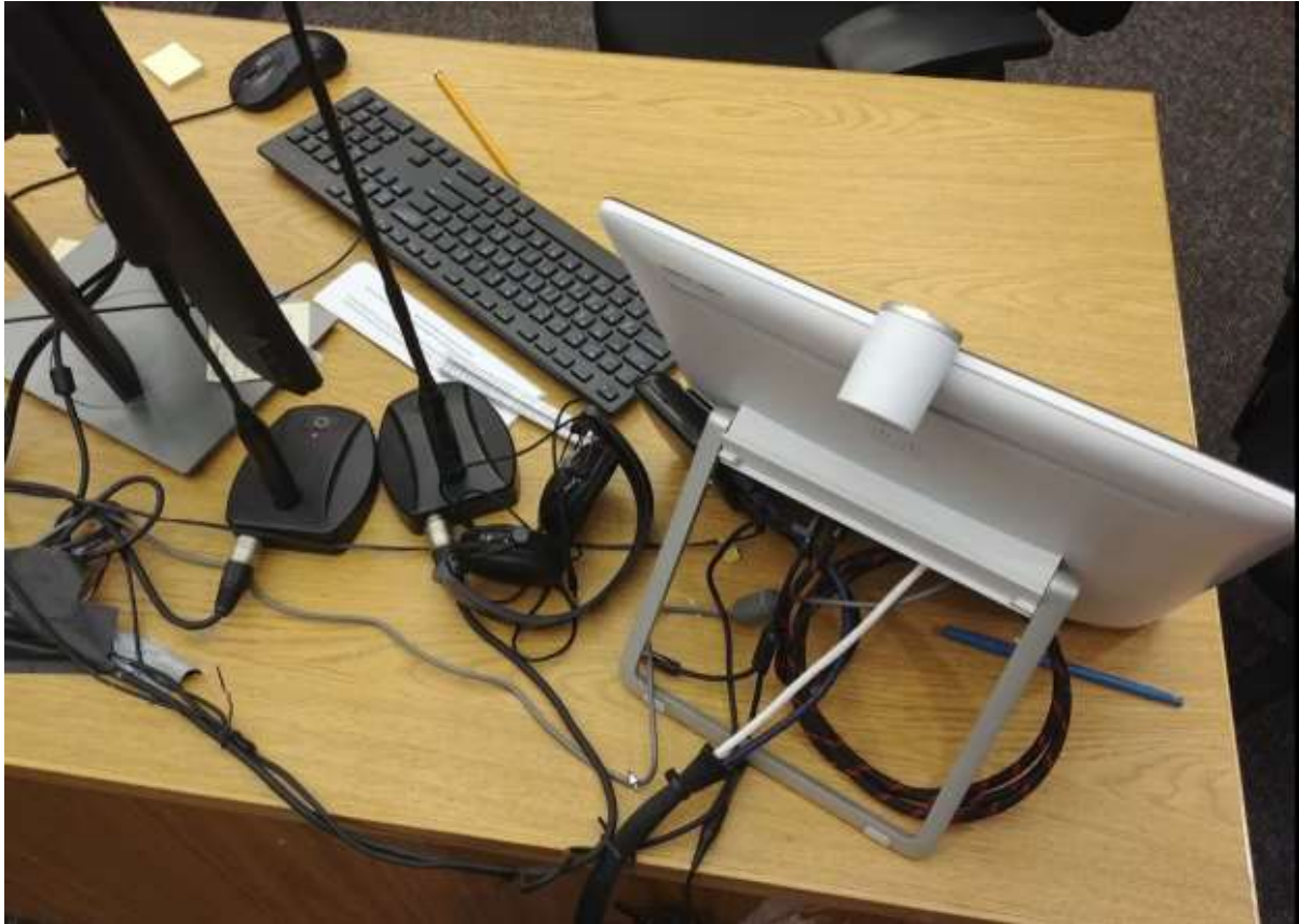
Detailed view of back of monitor. Equipment visible: HDMI receiver used to receive HDMI inputs from cameras, HDMI combiner used to combine HDMI signal and send to SX20.
