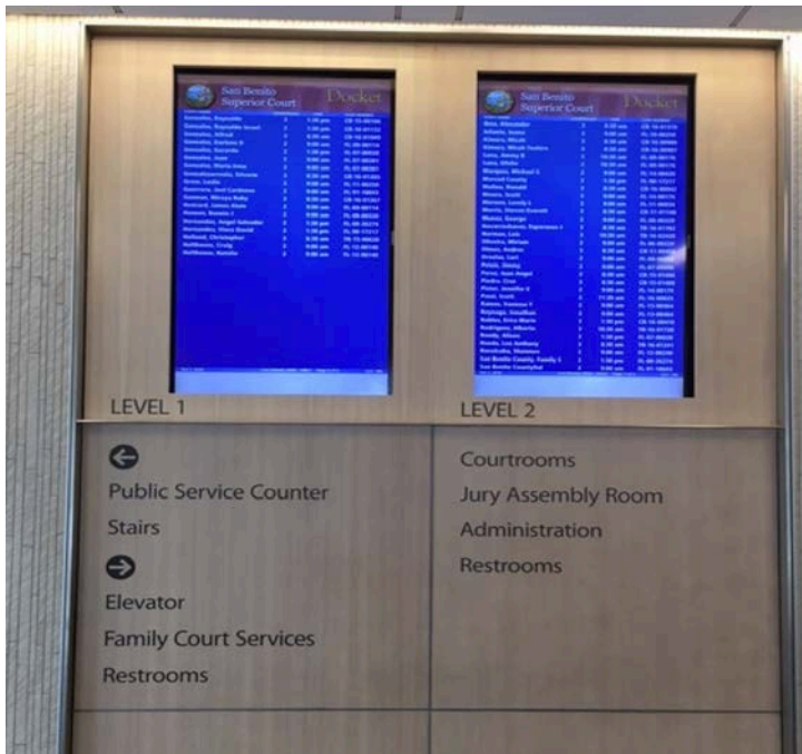
Figure 65 (left). Provided by San Benito. Illustrates the use of electronic signage together with static signage to provide information and directions.
