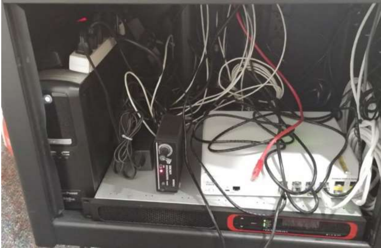
View of inside the media cart. Equipment from left to right: UPS, Biamp DSP, separate sound amplifier, Cisco networking switch.
