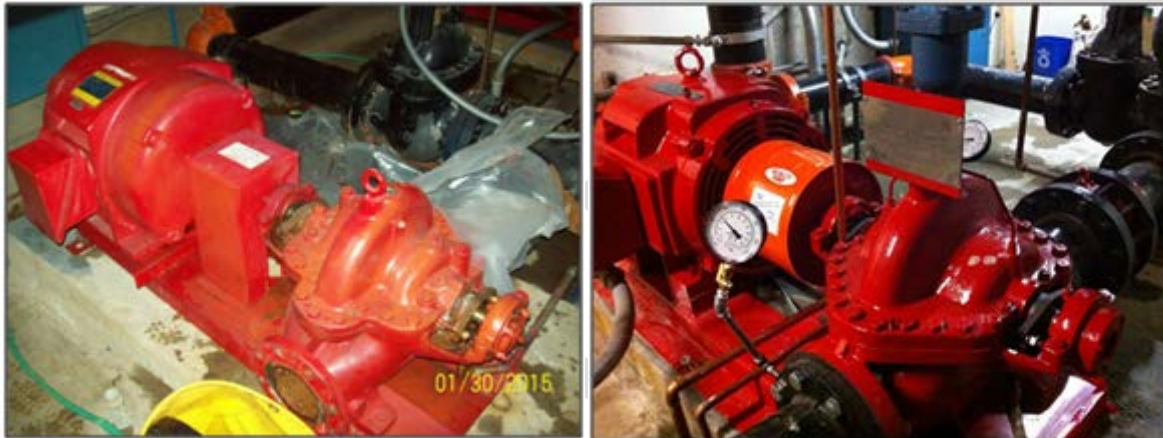
Above (left): One of the old fire pumps. Notice the evidence of leaking seals just above the date stamp on the main pump shaft. Above (right): A new fire pump, installed.
