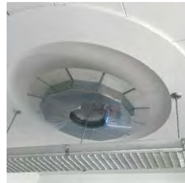
Figure 14. Recessed circular light fixture (ARG, 2022)
