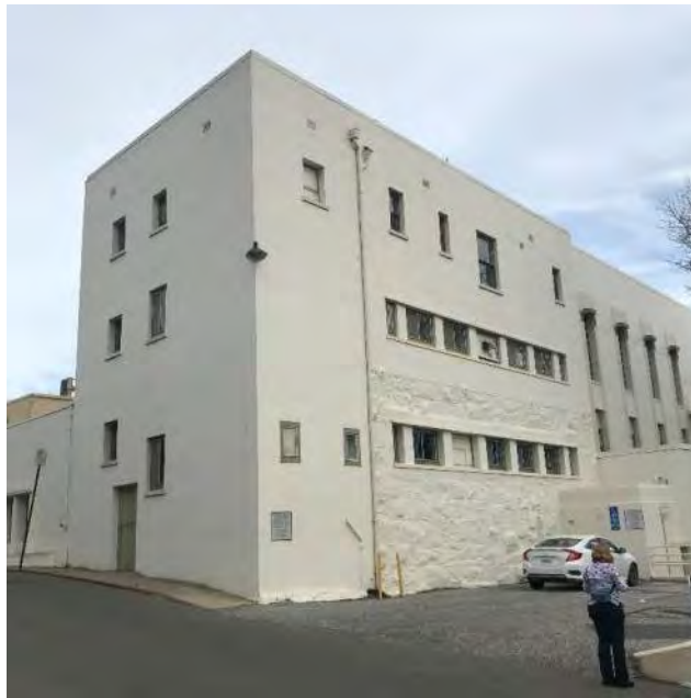
Figure 7. Granite wall at west side of north portion of the courthouse building, view southeast (ARG, 2022)
