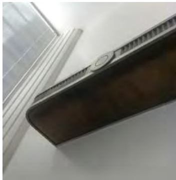
Figure 13. Detail at entry foyer including chrome lighting and vertically scored vertical embellishments (ARG, 2022)
