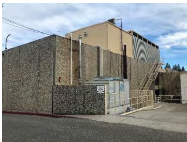
Figure 18. Annex, west façade, north portion, showing HVAC, penthouse, and exterior egress, view southeast (ARG, 2022)
