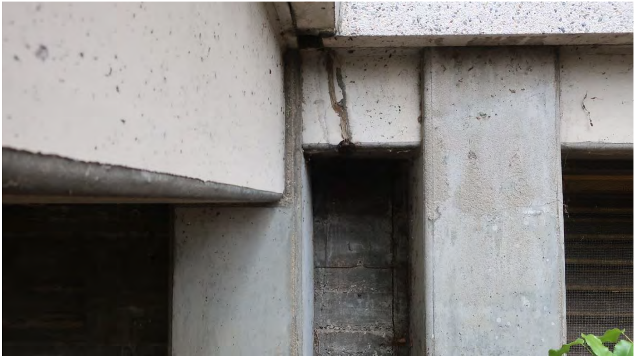
Photo 8: Cracked Concrete Beam and Wall at Annex Exterior
