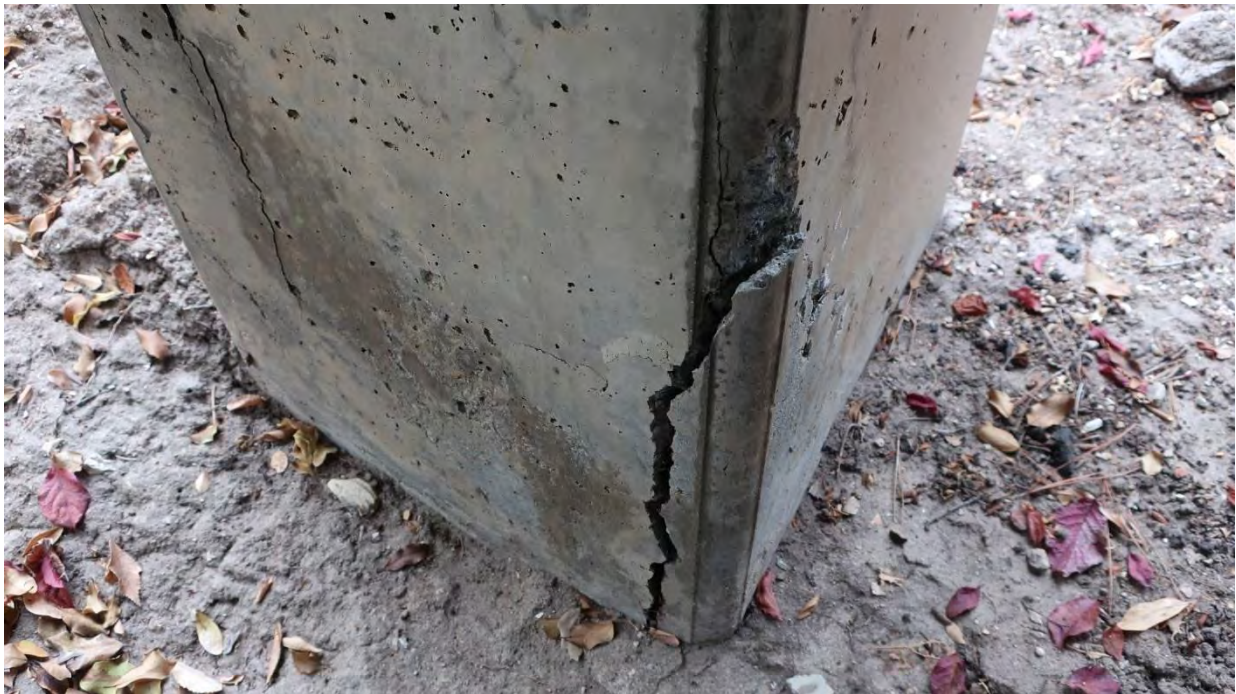
Photo 7: Spalled Concrete at Existing Column at the Annex
