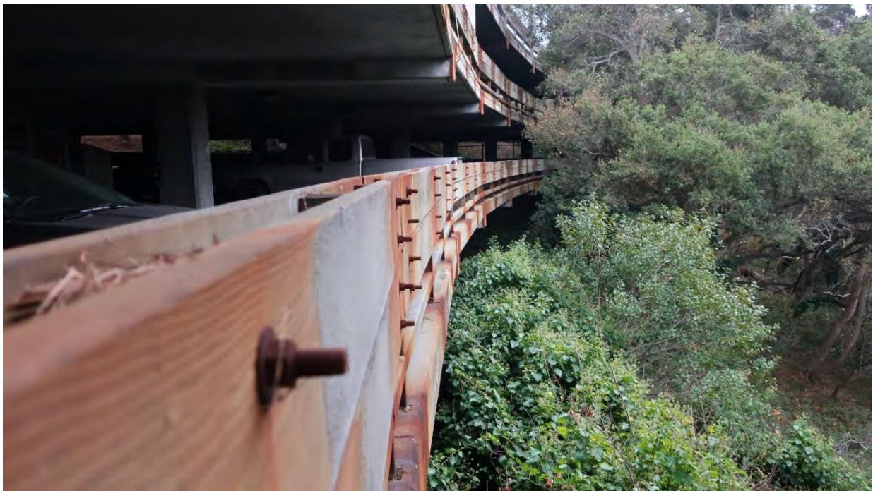
Photo 9: Corrosion at Parking Garage Guardrail
