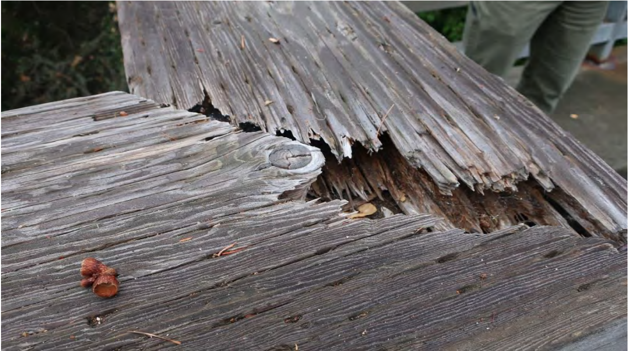
Photo 10: Deteriorated Wood at Parking Garage
