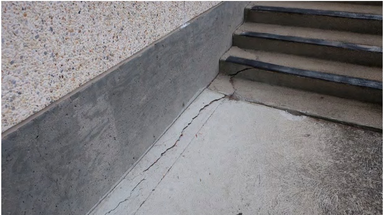
Photo 6: Cracked Exterior Sidewalk Slab at the Courthouse
