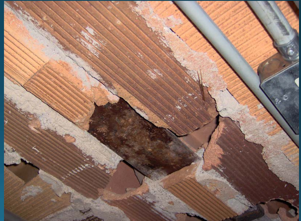
Basement ceiling-seismically unsafe
