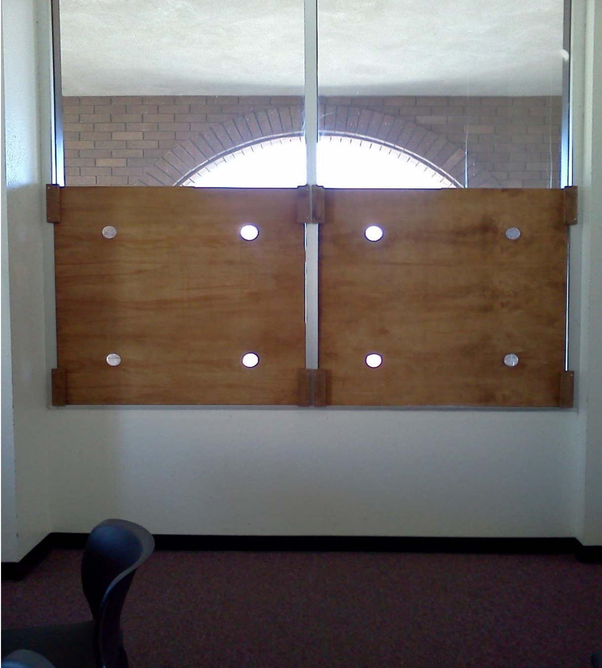
Plywood covering on windows in jury room where juveniles are held.
