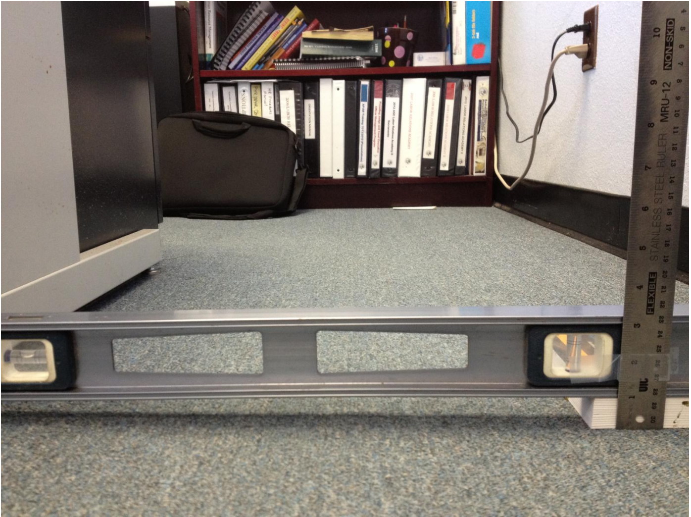
A six foot level showing nearly an inch slope in the floor of one office.
