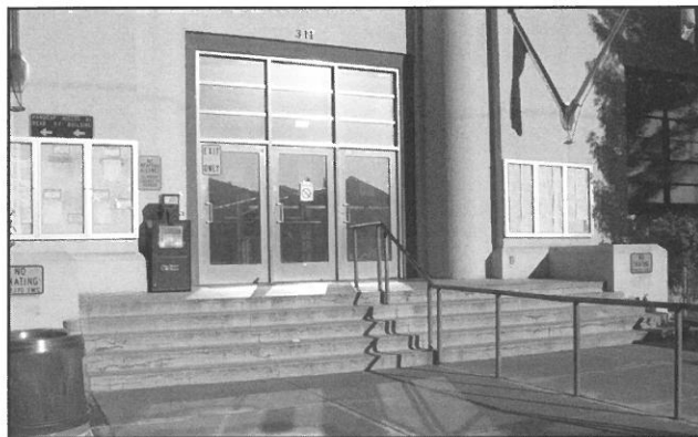
Front entrance to courthouse is not in compliance with ADA
