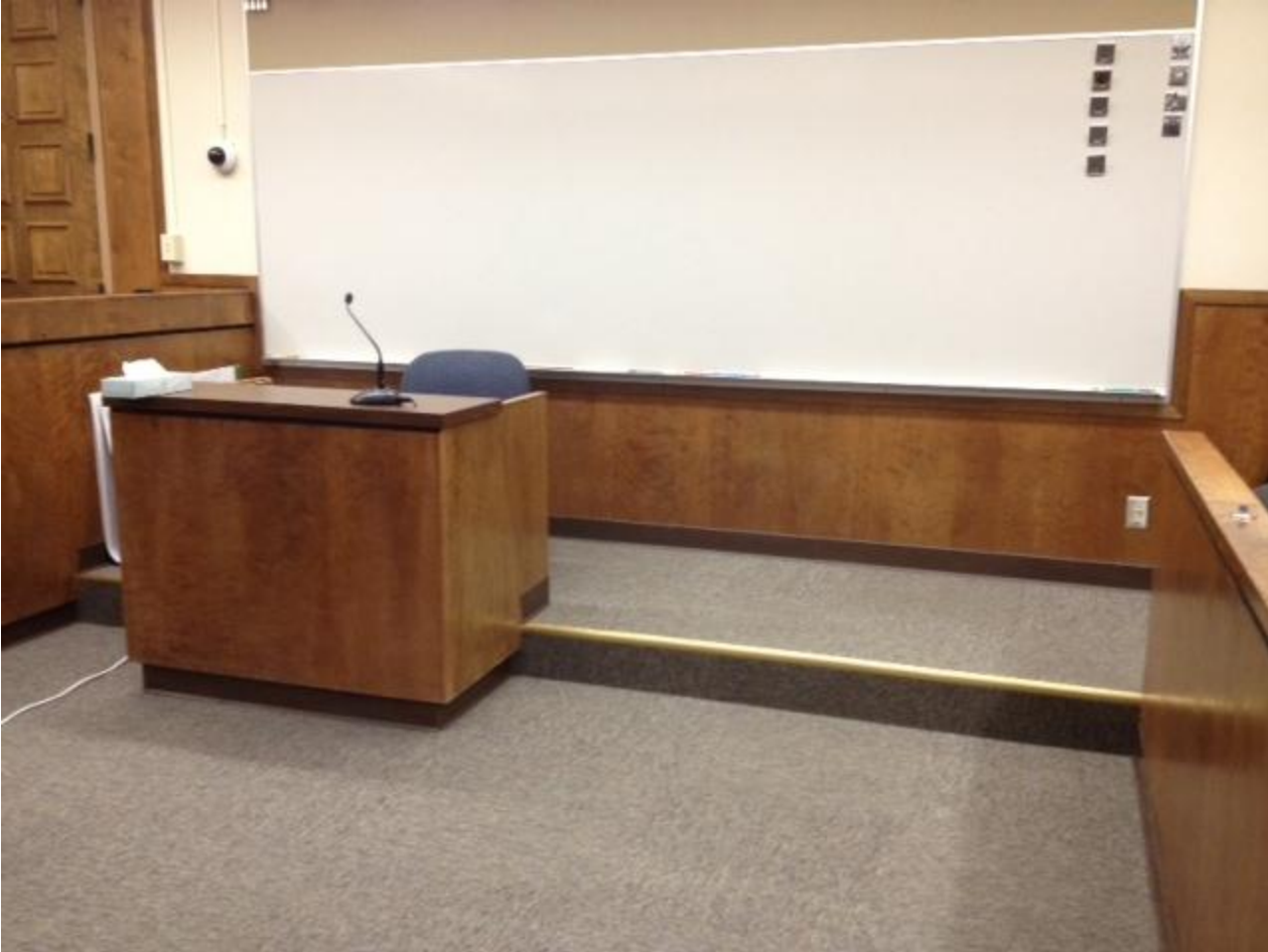
Witness box which is not ADA accessible.
