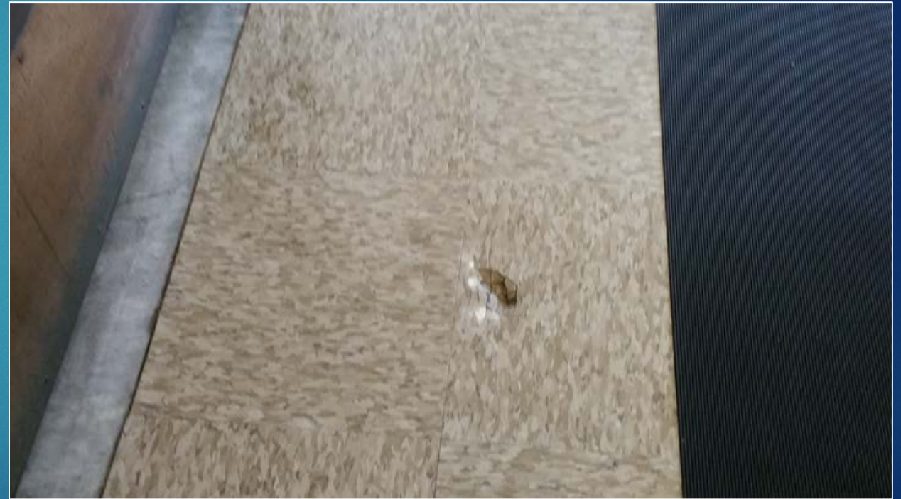
Sink hole in flooring tile outside public restroom
