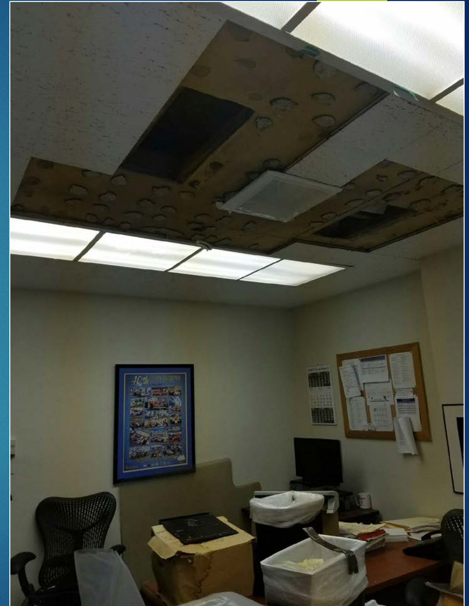
Water damage in DA's office from PD's restroom toilet, July 20, 2016
