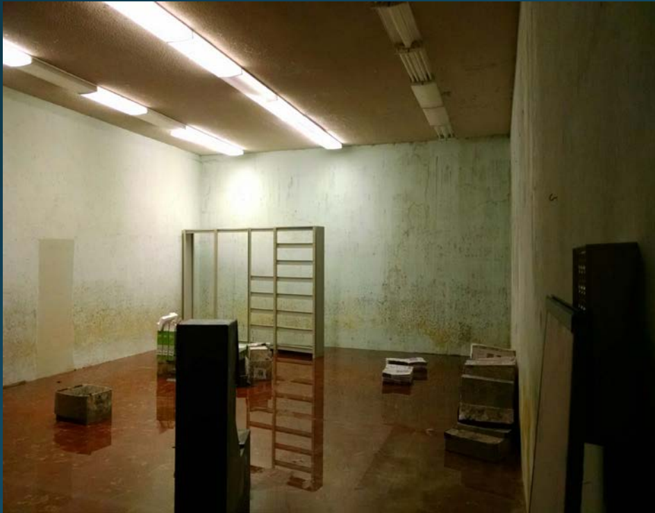
Leaky roof in vault
