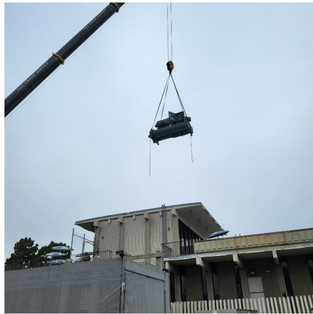
West Justice Center – HVAC (BMS)
