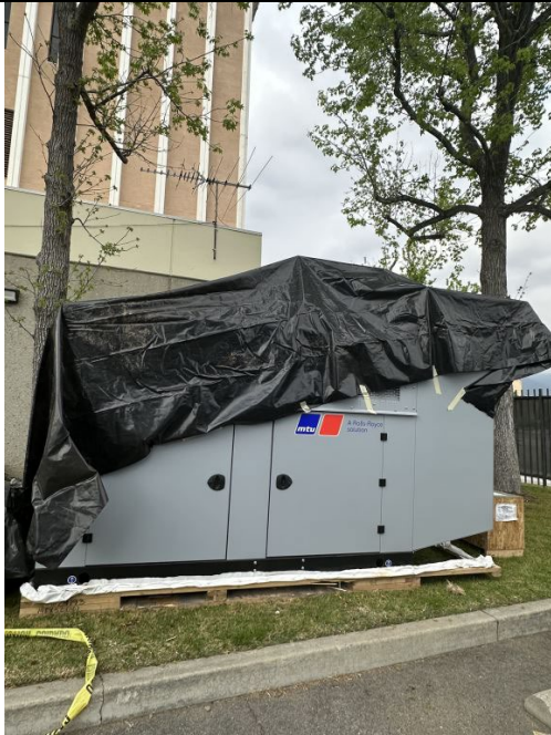
Pasadena Courthouse – HVAC (BMS)
